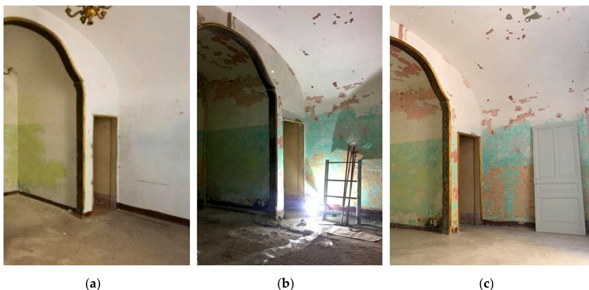
Figure 18. (a) Floor before starting work (room with alcove), (b) demolition of the floor and (c) new floor.
