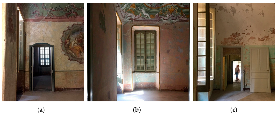
Figure 16. (a) Restoration of the walls of the second room, (b) restoration of the walls of the first room and (c) restoration of the walls of the room with the alcove.
