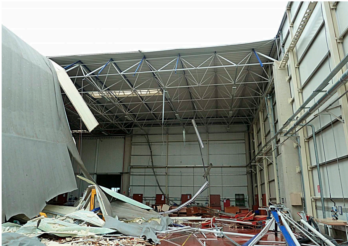
Figure 4. Damage to the roof's space truss system.
