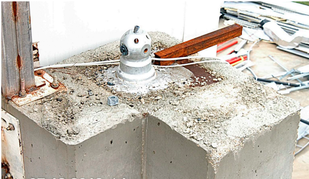
Figure 15. Damage on the support to which the space truss roof system was attached.
