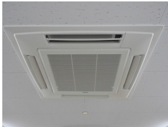
Figure 5. Example of the air conditioner under the ceiling.
