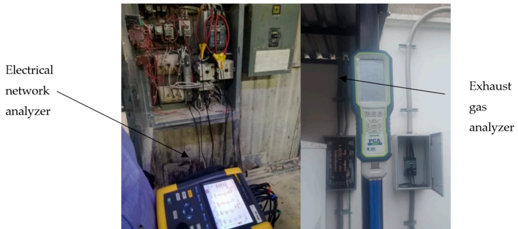
Figure 4. Connection of the network and exhaust gas analyzer.
