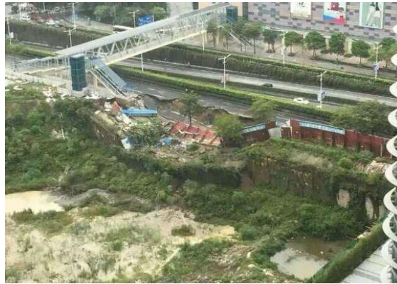
Figure 4. Collapse of an excavation in Foshan, China.
