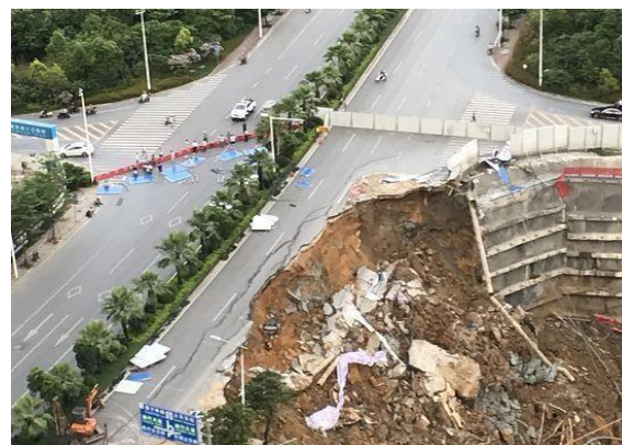
Figure 5. Collapse of an excavation in Nanning, China.
