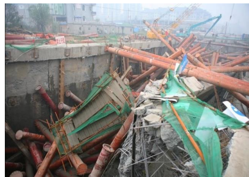
Figure 3. Collapse of Xianghu subway station in Hangzhou, China.
