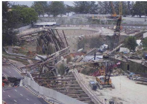
Figure 2. Nicoll Highway collapse in Singapore.
