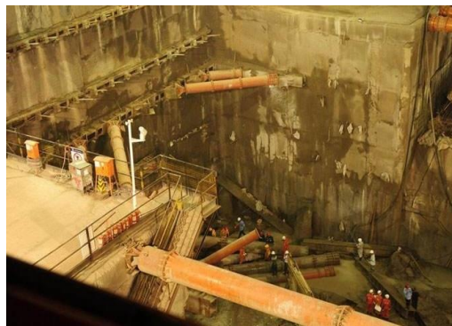
Figure 1. Strut failure of Shunyi Station in Beijing, China.
