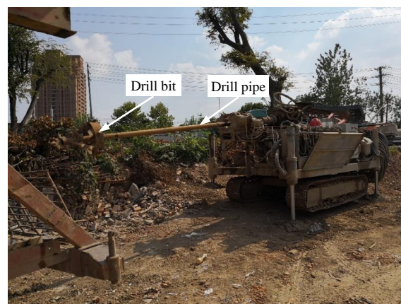
Figure 25. Photograph of the drilling machine used to drill holes for batter piles.
