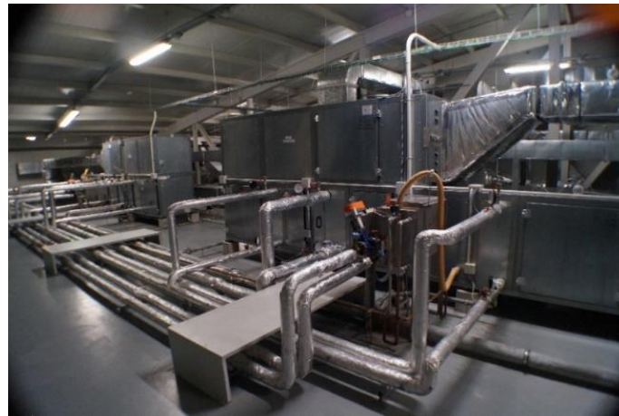
Figure 1. Heating, ventilation and air conditioning (HVAC) system of the surgical suite. In particular, Air Handling Units (AHUs) from OR2 and OR3.
