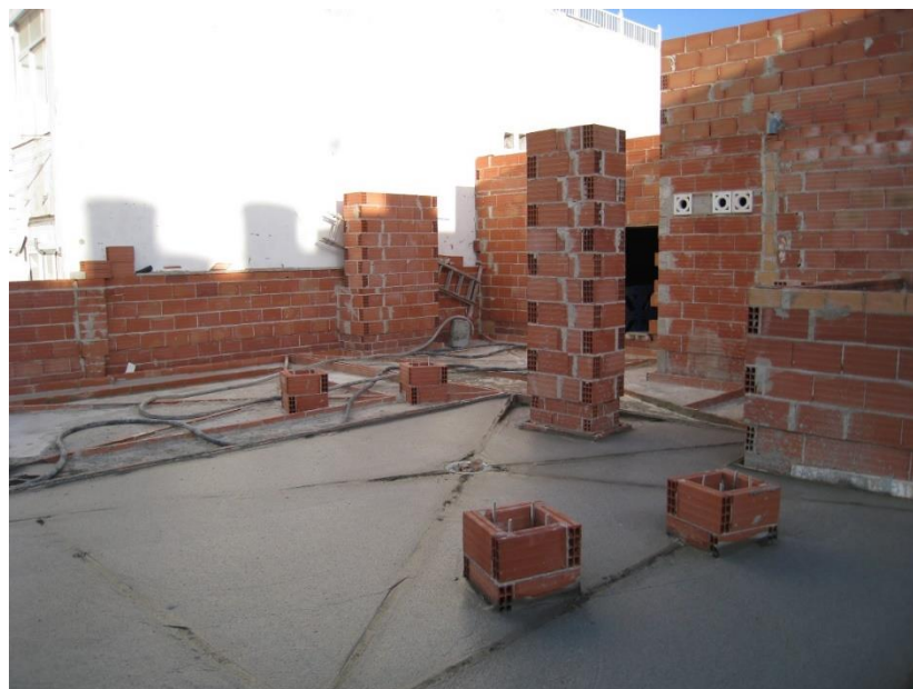
Figure 2. Image of the construction of walkable inverted flat roof of a housing block.
