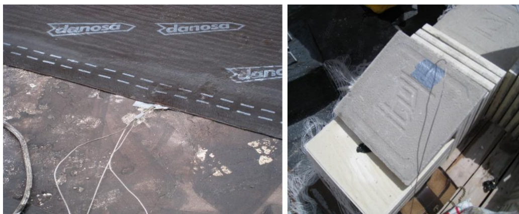
Figure 5. Installation of surface Type K thermocouple sensors on the apartment’s inverted flat roof.
