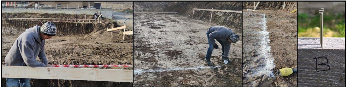
Figure 14. Construction twine and batter boards markings used for layout points positioning; obtained markings of the 4 methods of batter board stake-out (right).
