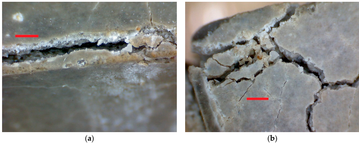
Figure 16. M3 after 285 days in the sulfate bath: (a) cracking on the longitudinal edge of a specimen; (b) a network of cracks in the corner of a specimen; the red line indicates a length of 1 mm.
