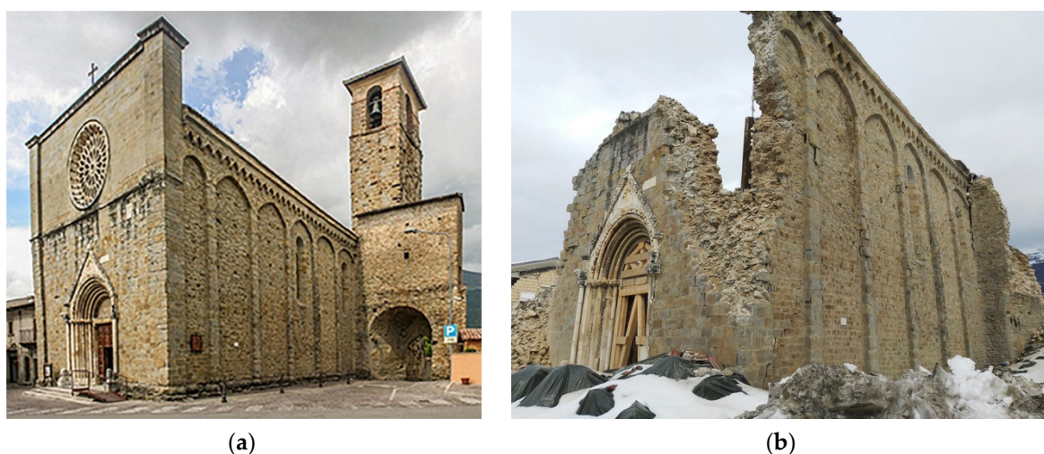
Figure 1. St. Agostino church in Amatrice before (a) and after (b) the seismic earthquake swarm of 2016 in Central Italy.
