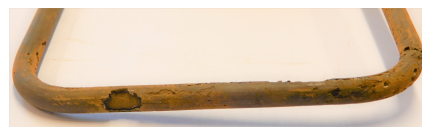
Figure 12. Picture of the stirrup of sample AE-2 after removal and cleaning at the end of the accelerated corrosion test.
