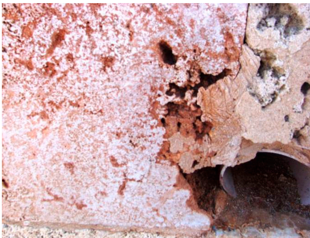
Figure 10. An efflorescence of kurkar siding in the Panorama sea walls. Captured by the author on 27 November 2018.
