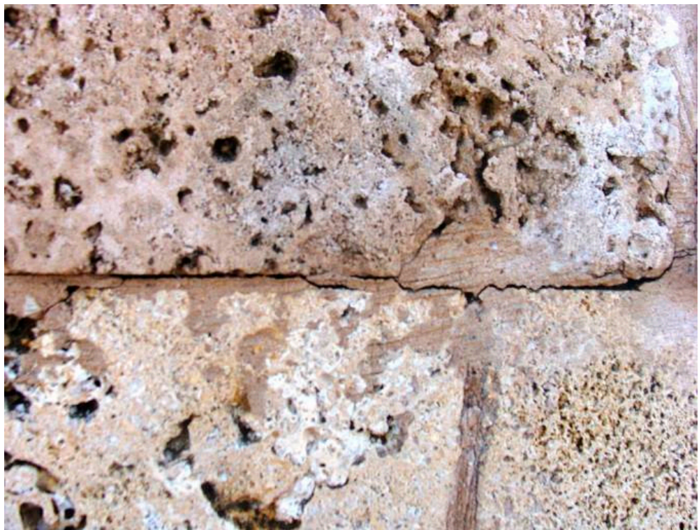
Figure 7. Weathering out of stone components in the Panorama sea walls. Captured by the author on 27 November 2018.
