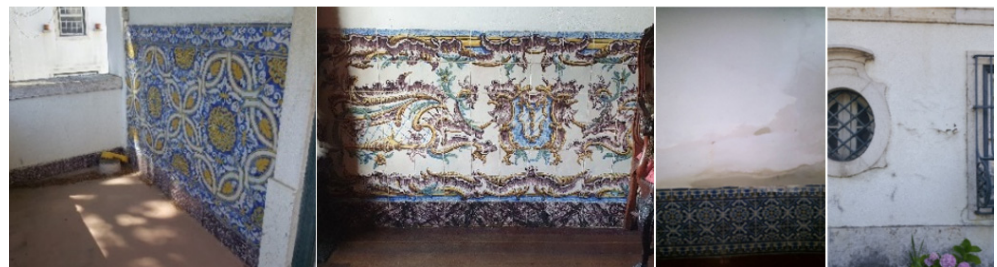
Figure 10. Decorative ceramic tiles applied to wall surfaces and detection of deterioration.
