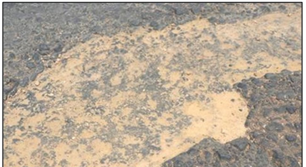
Figure 24. Stripping of surfacing (double seal with an elastomer modified binder) due to a contaminated binder (December 2018), resulting in little damage to an exposed NME stabilised base-layer after 2 months of traffic in the rainy season (in situ material originally of quality CBR > 10 @ 93% mod AASHTO) (Gauteng Province, South Africa).
