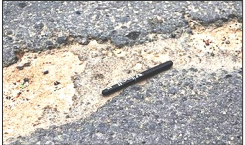
Figure 23. Stripping of asphalt (35 mm) (December 2019) due to placement of the asphalt in wet conditions (rain)—anionic NME stabilised base has been exposed for 2 months during the rainy season (Original material quality: CBR 15 to 25 @ 93% mod AASHTO) (Mpumalanga Province, South Africa).
