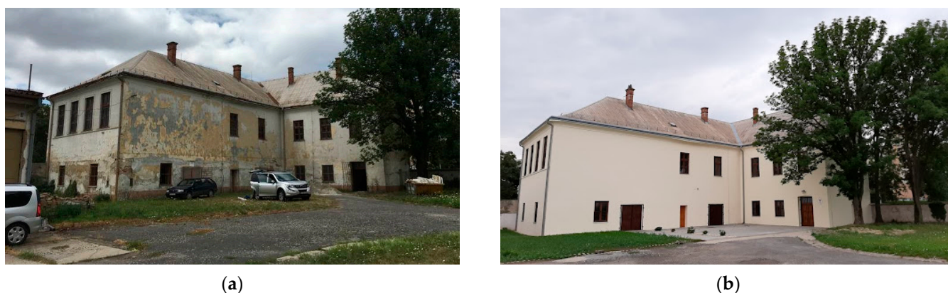
Figure 5. View on the state of building (a) before and (b) after recovery.
