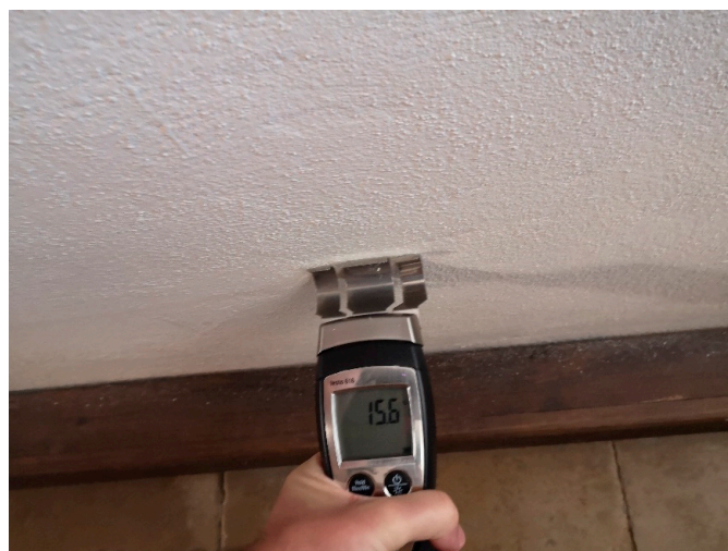
Figure 7. A picture representing the moisture rate of the structure.
