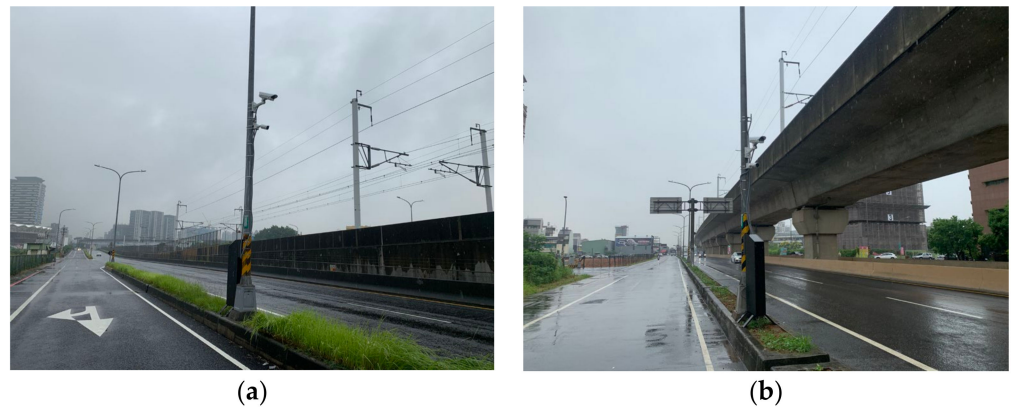
Figure 18. Installation of the LED roadway lighting system: (a) Sect. 3 of Gaotie South Road; (b) Sect. 5 of Gaotie South Road.
