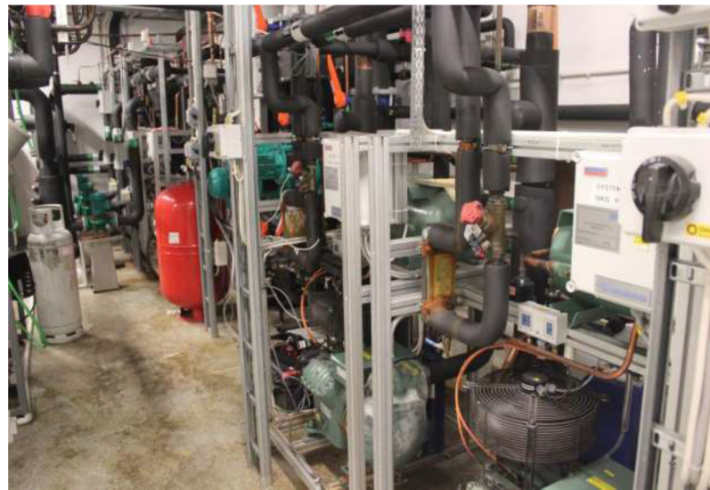
Figure 2. Supermarket refrigeration system used in this study.
