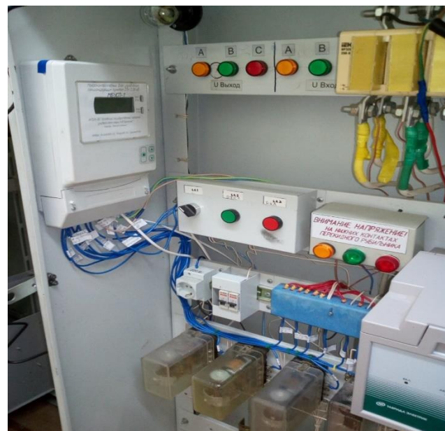
Figure 3. Inside view of SU combined with electricity metering and power quality control.
