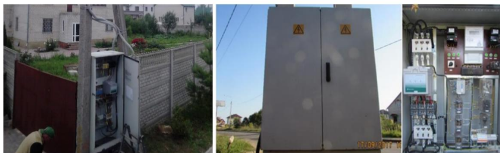
Figure 1. Photos of sectionalizing units installed in Orel electrical networks [37].
