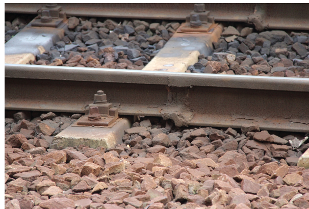
Figure 7. Thermite weld joining two rails with different profiles (50E5, UNI-50, on the right and 60E1, UNI-60, on the left).
