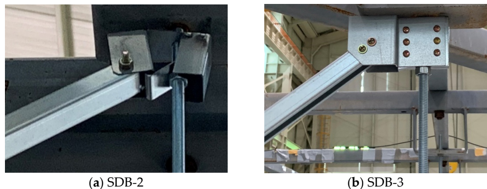
Figure 11. Brace-hanger bolt connection, Test 8 (2.16 g), (a) yield of the SDB-2 connection and (b) SDB-3.
