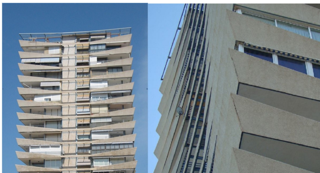
Figure 3. State of the building's façades and parapets in 2010, before its refurbishment.
