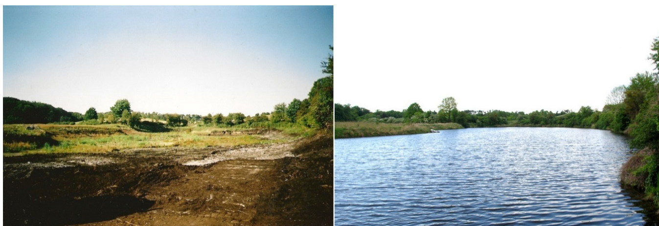
Figure 3. Part A of pit lake under construction (left) and one year after works (right).
