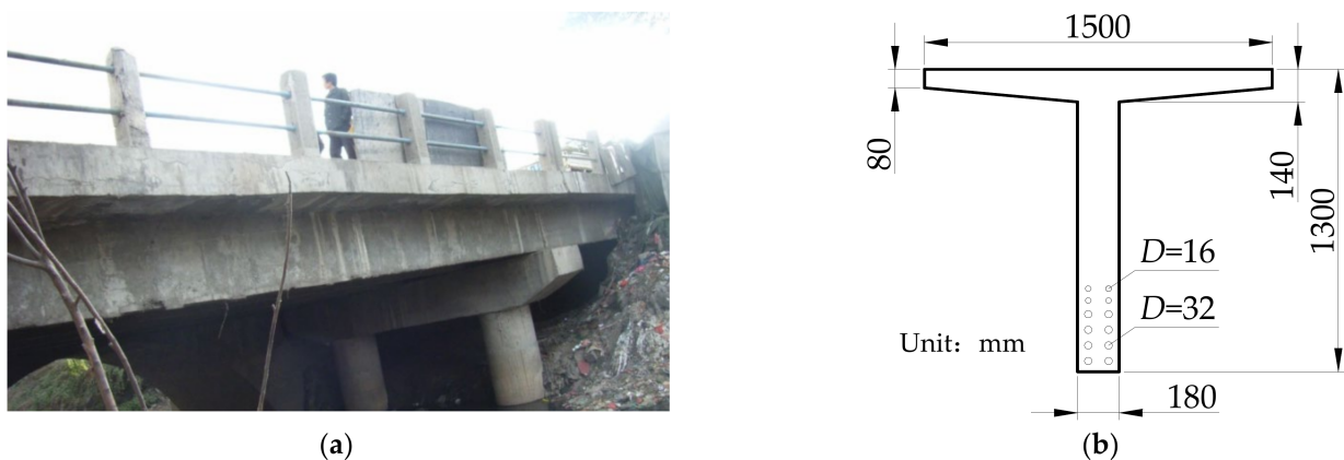
Figure 3. Appearance of typical simply supported T-beam bridge: (a) profile of Xiaobai Bridge; (b) cross-sectional dimension drawing of T-beam.
