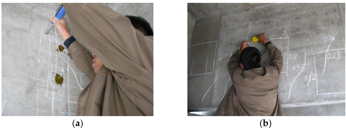
Figure 4. Field test diagram: (a) detection of concrete strength; (b) detection of concrete cover thickness.
