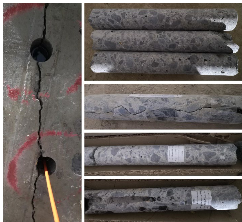
Figure 4. Concrete crack and concrete cores.
