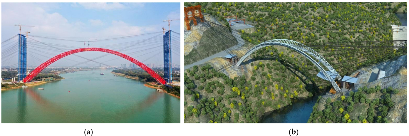
Figure 1. Cable lifting construction of large-span arch bridges: (a) Pingnan Third Bridge; (b) Jinghe Bridge.
