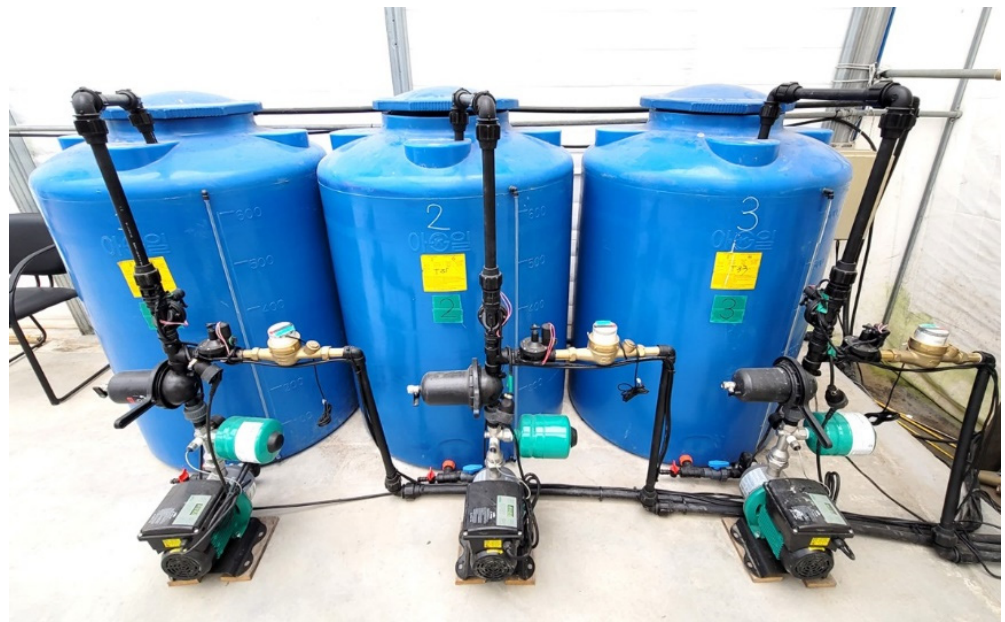
Figure 4. The photo of the pressure pumps and solenoid valves in the experimental field.
