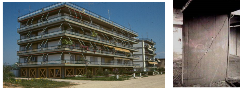
Figure 2. Temporary wooden story. Damaged shear wall at the soft story.
