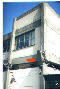
Figure 4. Damaged short columns from the interaction of unreinforced masonry infills (UMI), built within the bay of an RC frame structure, with the adjacent RC columns.
