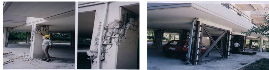
Figure 3. Damaged columns at the soft-story and temporary steel shoring.
