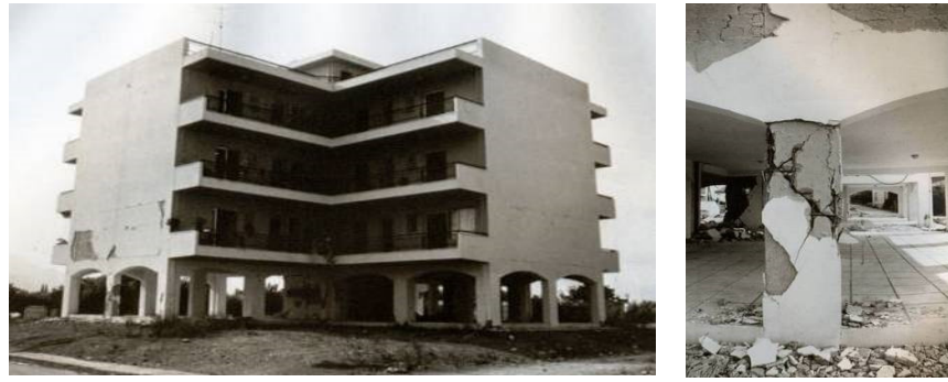
Figure 1. Damaged columns at the soft story.
