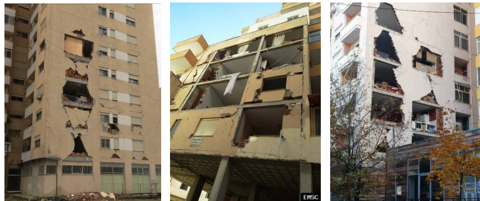
Figure 9. Out-of-plane collapse of unreinforced masonry infills (UMI) panles from RC frame structures due to earthquake excitation.
