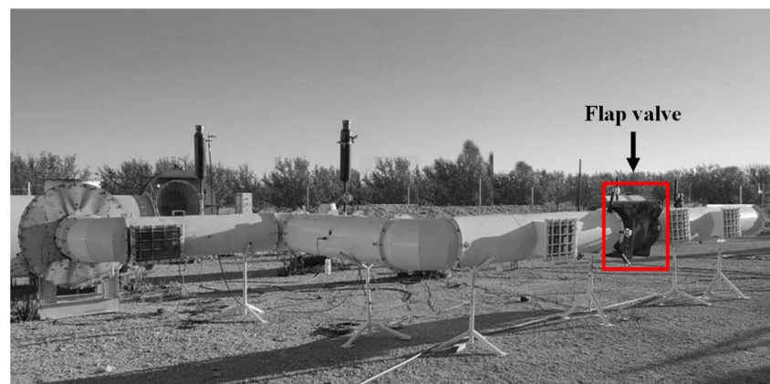
Figure 2. Test setup for a DN500 flap valve mounted at a distance of 10.2 m measured from the 1 m 3 vessel, in a duct with three short radius bends (R/D = 0.6).
