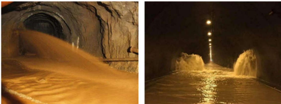
Figure 4. Tunnel water inrush site and water pressure test chart.
