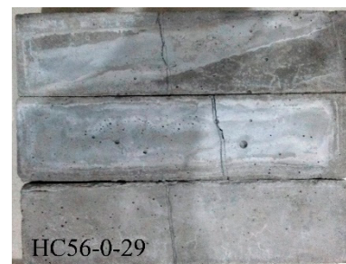
Figure 4. Failure pattern of the control specimens.
