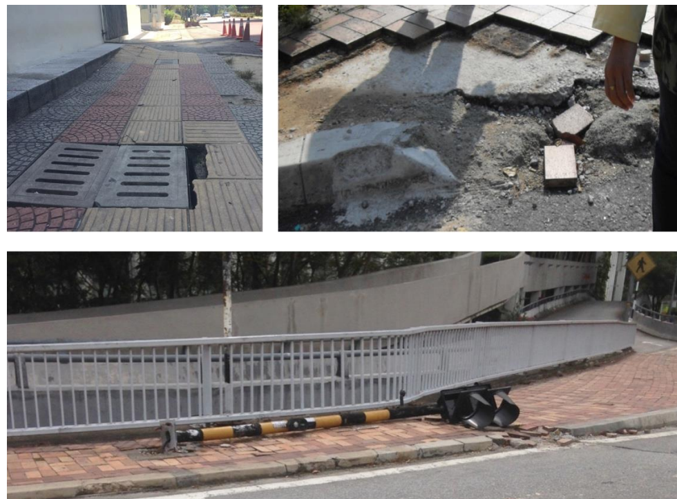
Figure 4. Damaged pedestrian paths in KL, Malaysia.
