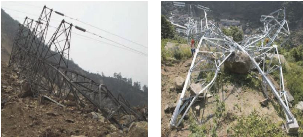
Figure 1. Collapsed transmission towers in China caused by the Wenchuan earthquake [30].
