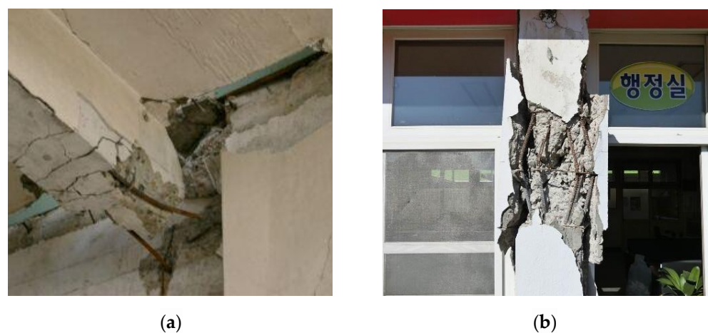
Figure 3. Corrosion of RC beams and columns damaged during earthquakes. (a) the 2004 Niigata-ken Chuetsu Earthquake in Japan and (b) the 2017 Pohang Earthquake in Korea.
