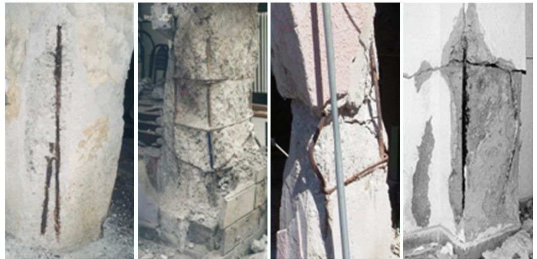
Figure 2. Corrosion of RC members damaged during the 1999 Izmit Earthquake in Turkey.
