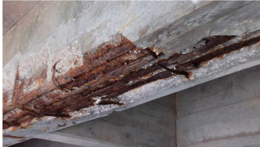
Figure 1. Structural performance deterioration of a reinforced concrete (RC) structure due to reinforcement corrosion.
