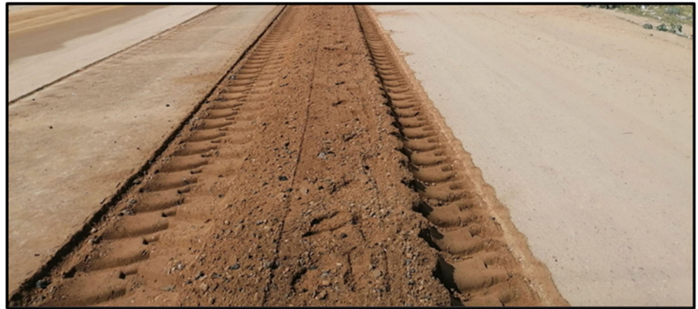
Figure 9. Uniform visual appearance of a uniform mix of granular material with an anionic NME stabilising agent in construction water as mixed with a recycler.
