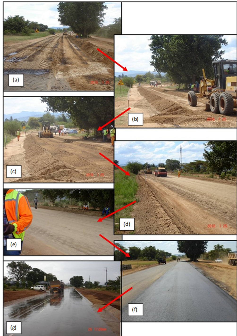
Figure 11. Resolving uneven distribution of a NME stabilising agent (Figure 10): (a–c) Through the remixing of the road pavement layer using a conventional grader; (d,e) compaction of the remixed layer showing the uniformity achieved with the grader; (f) primed surfacing of the layer remixed using a grader; (g) finished road with surfacing on the section of road with the original uneven distribution of the stabilising agent (Figure 10).
