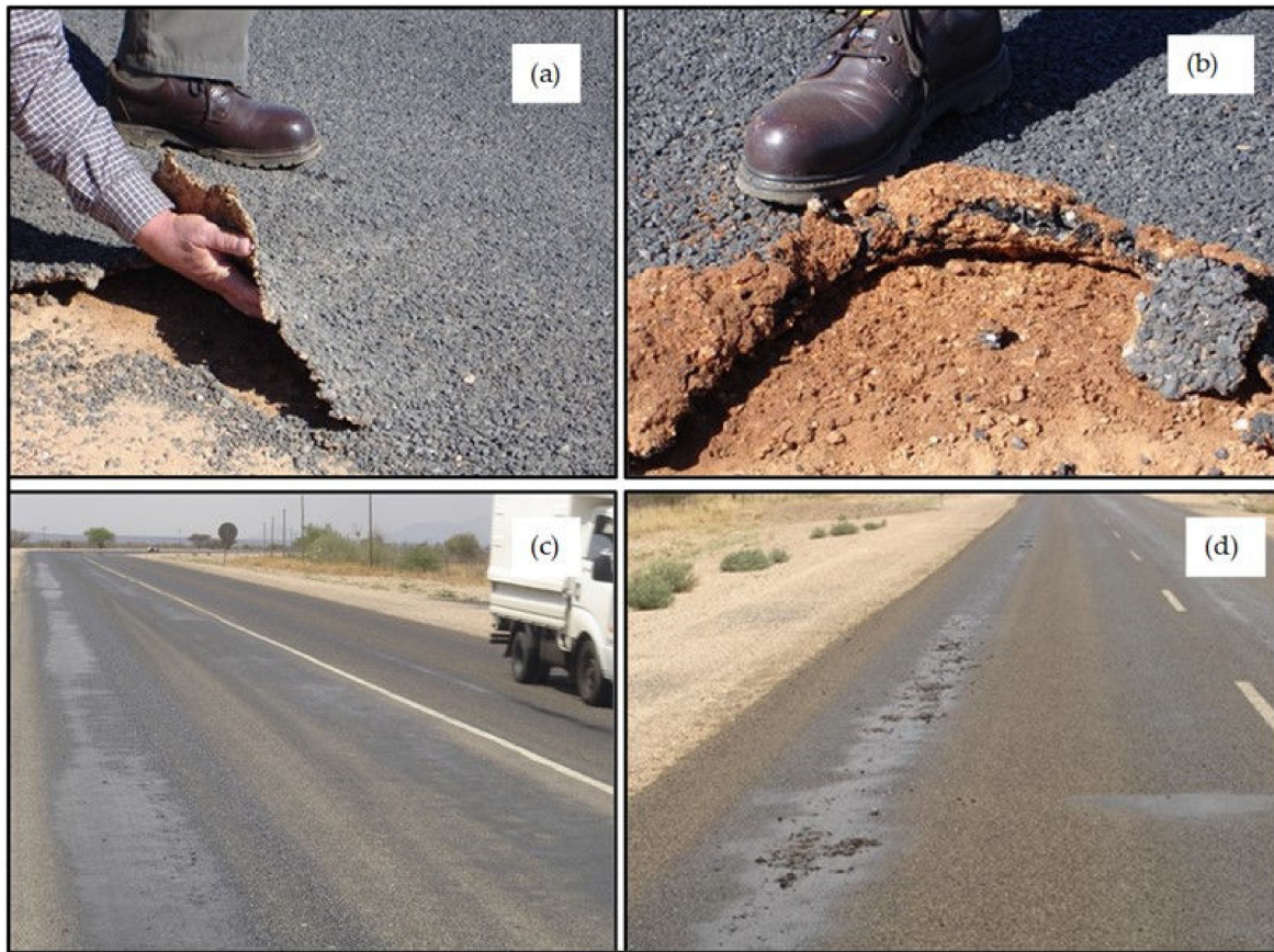
Figure 16. (a) Detachment of the surfacing from the base layer; (b) moisture collecting under a surfacing that inhibits the escape of moisture fumes leading to the conditions shown in (a); (c) punching of the surfacing into the base layer; (d) failure resulting from the punching of the surfacing into the base layer.
