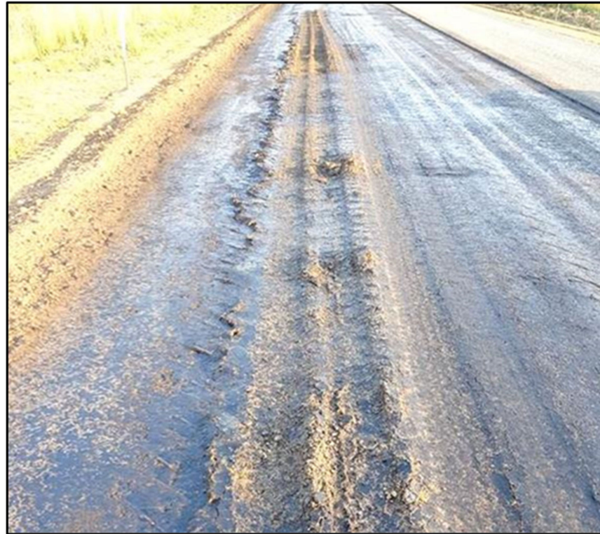
Figure 5. Severe movement of the NME stabilised layer, which is indicative of layer thicknesses that do not comply with specifications. The NME stabilising agent was added to a very thin layer (50 mm) instead of the specified 150 mm.
