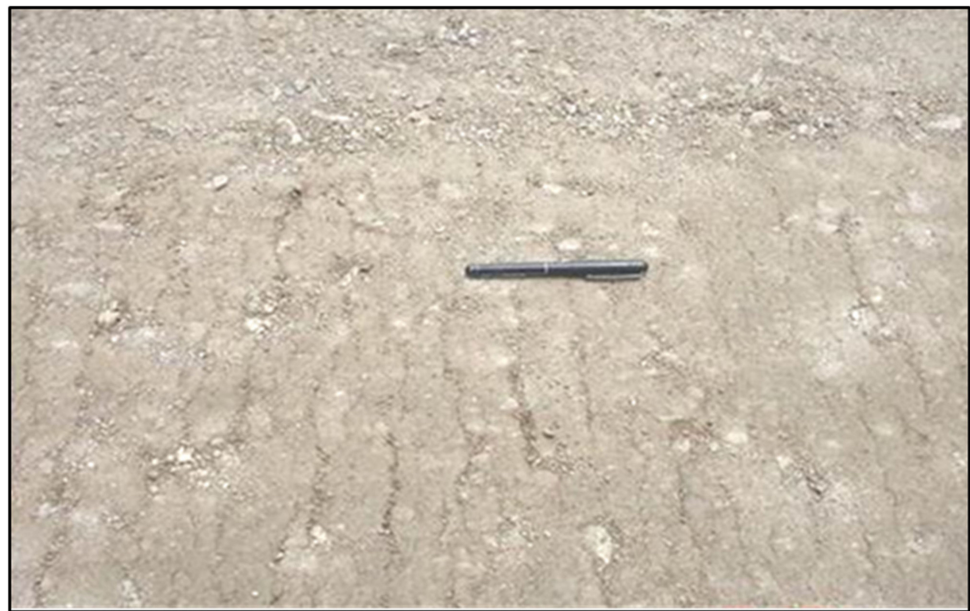
Figure 4. Appearance of small cracks on the surface directly behind a smooth-drum roller which are indicative of moisture conditions in the construction layer that are too low to achieve good compaction.
