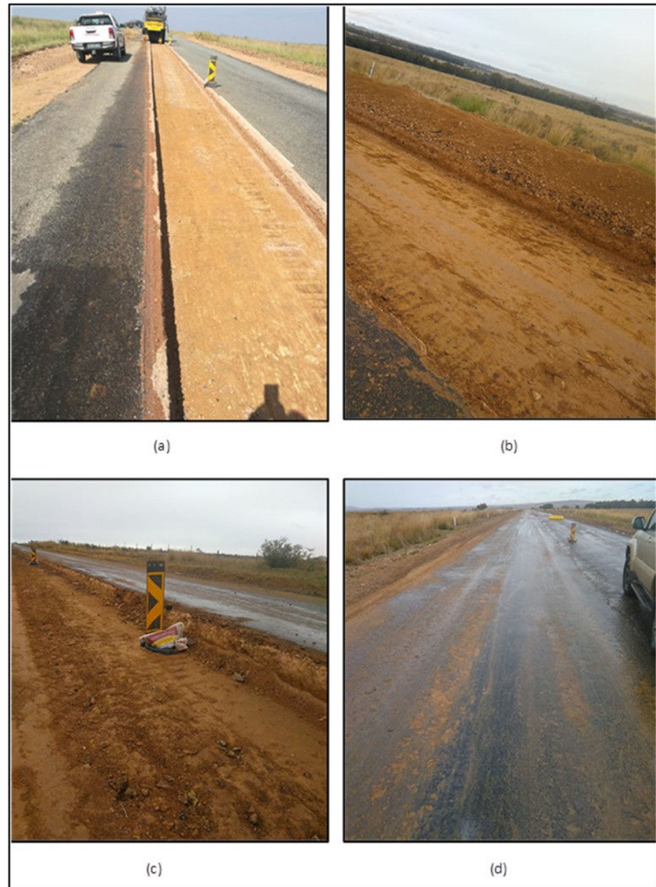
Figure 17. (a) Milling of existing base and sub-base layers to be stabilised using an anionic NME stabilising agent; (b) stockpiling of material next to the road; (c) depth of milling and new roadbed to be compacted; (d) reintroduced sub-base and base separately stabilised using an anionic stabilising agent.
