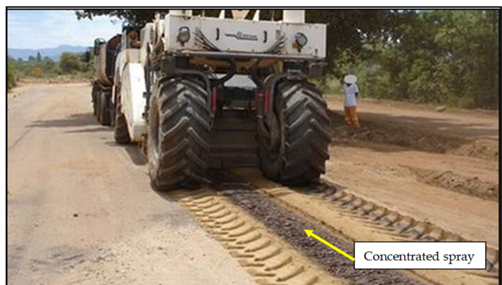
Figure 10. Uneven distribution of an anionic NME stabilising agent in construction water behind a recycler, caused by blocked spray nozzles of the recycler.
