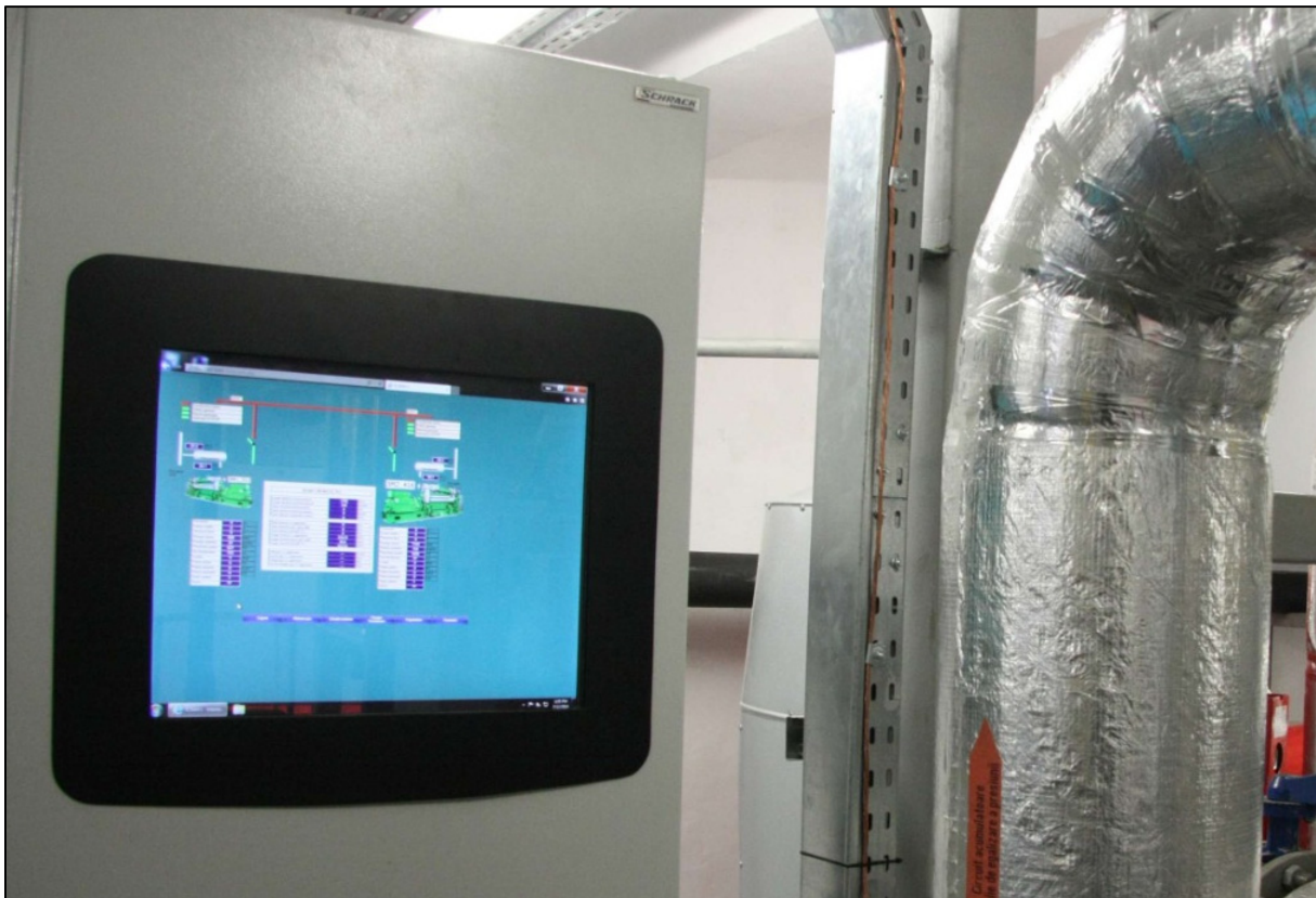
Figure 8. The PLC that controls and monitors the cogeneration plant.
