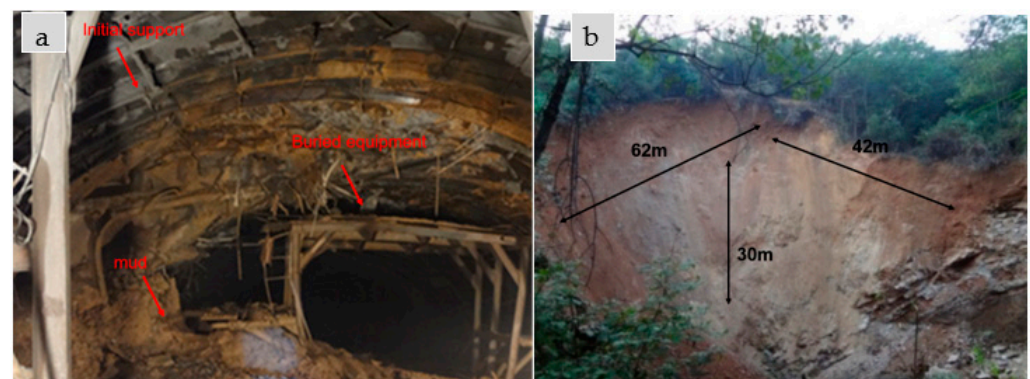
Figure 2. Partial mud inrush disasters and the collapse pit. (a). Mud inrush disaster in tunnel. (b). Collapse pit at the mountain peak.
