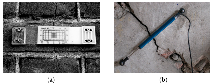
Figure 2. Monitoring of cracks employing: (a) plastic Tell-Tale crack meter, and (b) an LVDT sensor (from [48]).
