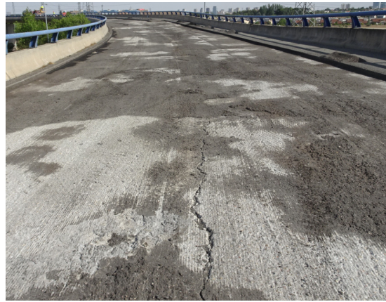
Figure 5. Longitudinal cracks in the deck's upper face.
