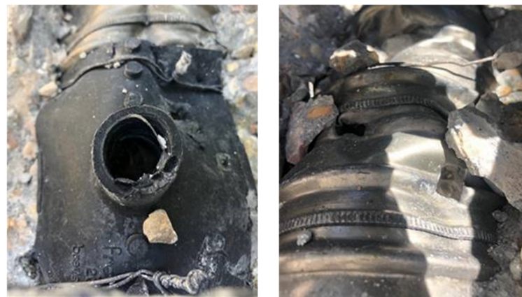
Figure 11. Lack of connection between venting pipe and prestressing sheath (Colmenar Bridge).
