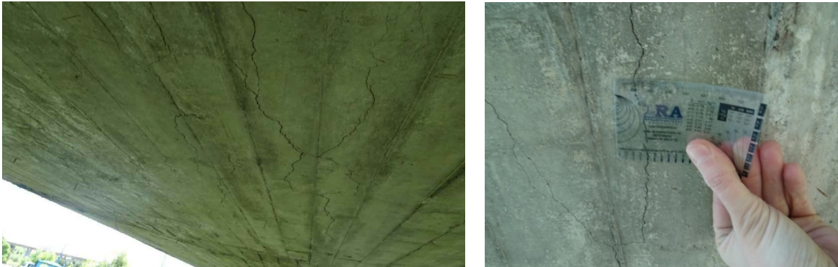
Figure 3. Longitudinal cracking on the bottom surface of the deck.
