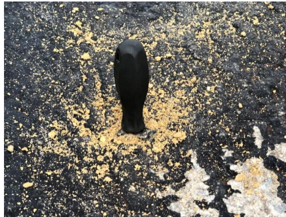
Figure 8. Venting pipes check to verify the clogged conditions (see the handle of the screwdriver inserted into the hole).
