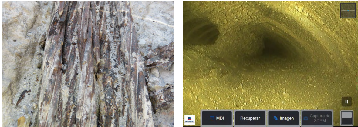
Figure 10. On the left, corroded cords and broken wires; on the right, unusual grout consistency with foam formation.
