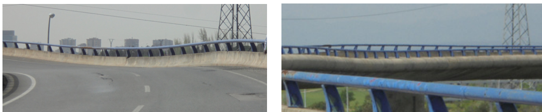
Figure 4. Marked deflections in spans # 5 and # 8 of Nudo de Colmenar structure.
