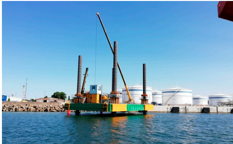
Figure 2. Construction work carried out close to navigational channel in Klaipeda port [own picture].
