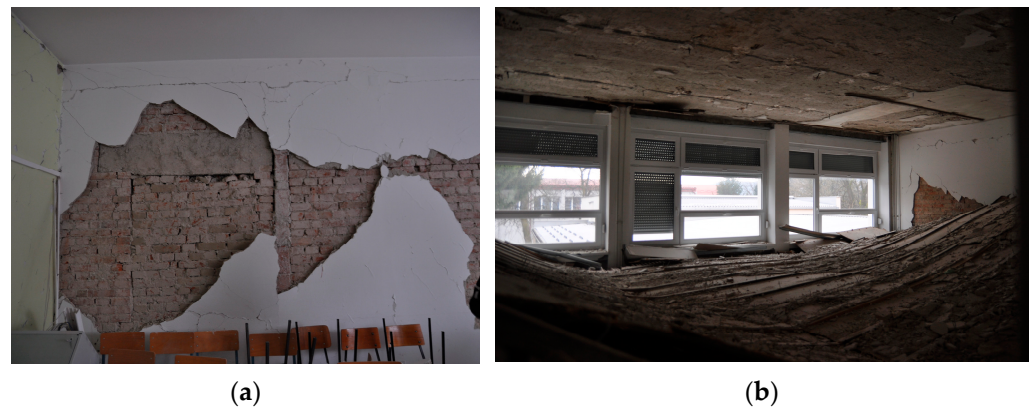
Figure 4. Observed damage on (a) the partition wall and (b) the ceiling.
