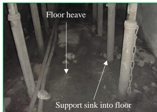
Figure 4. Damage diagram of the floor heave of the gob-side entry retaining roadway.
