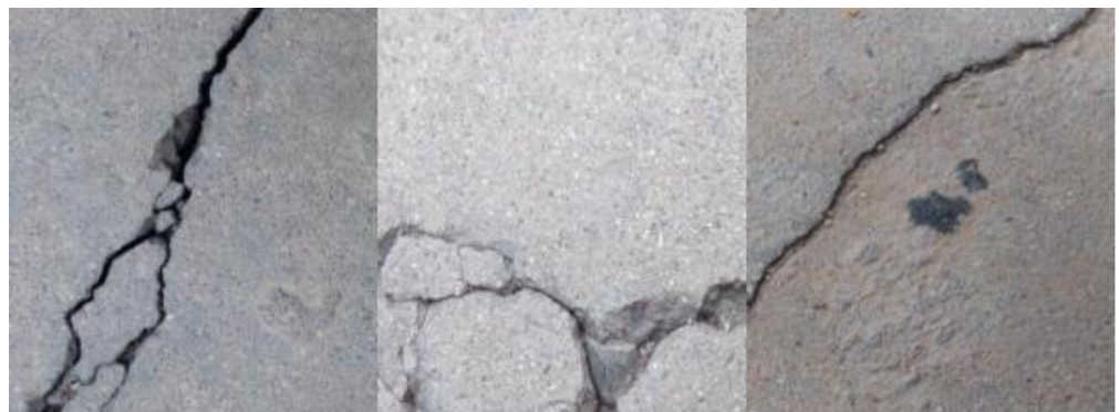
Figure 10. Examples of crack images.
