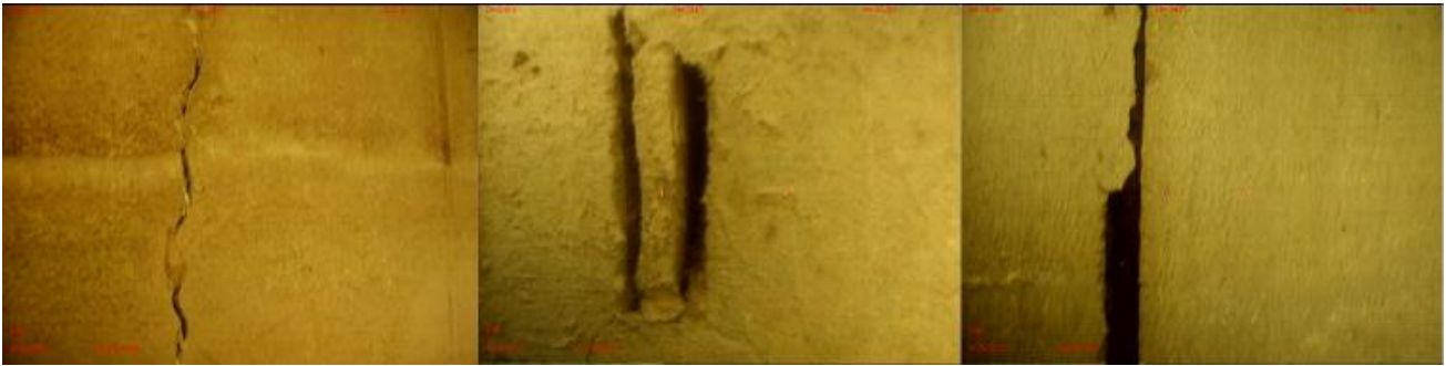
Figure 9. Examples of underwater dam concrete crack.
