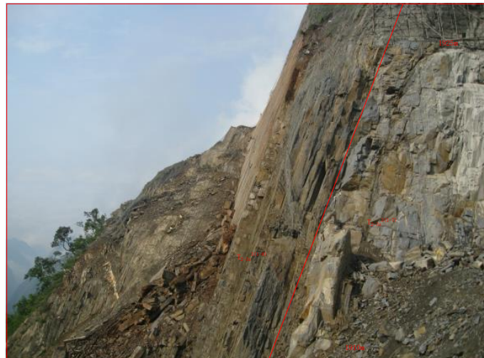
Figure 5. Slipping along interlayer.
