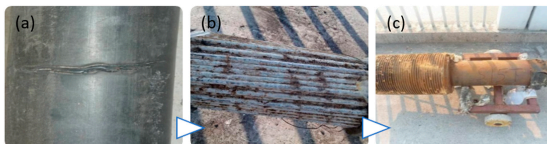
Figure 4. Typical cable diseases of a cable-stayed bridge: (a) PE sheath cracking, (b) steel wire corrosion, (c) anchor cup corrosion.
