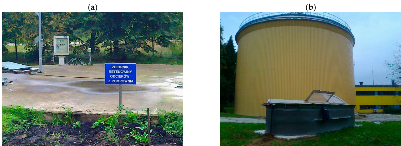
Figure 3. LF-DSS storage tank (a), enclosed digester and chamber filter press building, with the H-PBR in the foreground (b).
