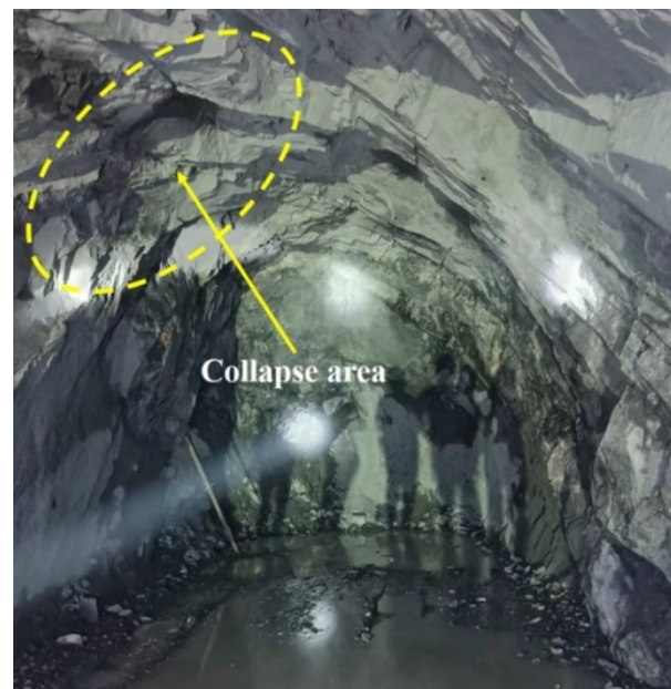
Figure 14. Collapsed zone of the tunnel at the field site.
