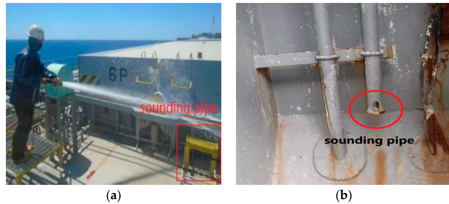
Figure 10. No.6 cargo hold sounding pipe. (a) Sounding pipe deck part; (b) Sounding pipe bottom part.
