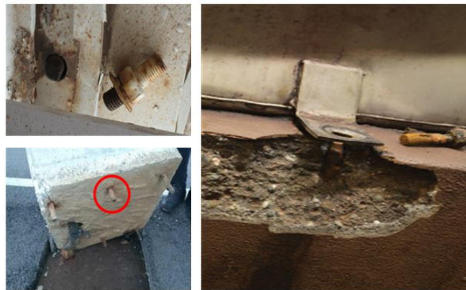
Figure 1. Damage to protrusion concrete caused by overturning under earthquake conditions.
