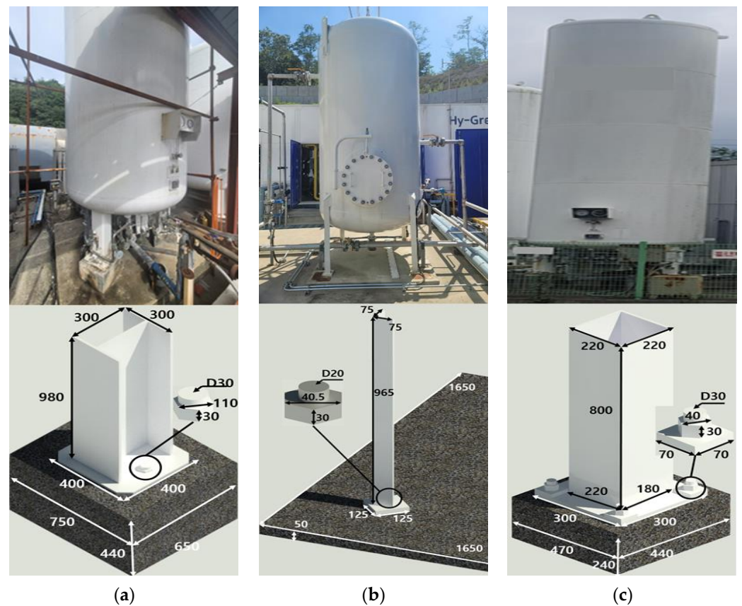
Figure 3. The configuration and support system of the target structures installed in each region (unit: mm): (a) Gangneung, (b) Samcheok, and (c) Ulsan.
