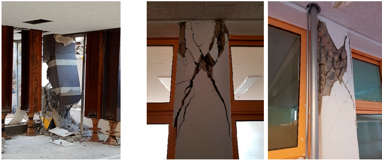
Figure 1. Shear damage of R/C buildings in the 2017 Pohang Earthquake [1].
