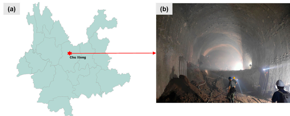
Figure 3. Location of CYWDP. (a) Location of Chuxiong in Yunnan province; (b) condition of the work face in the RBSR tunnel.
